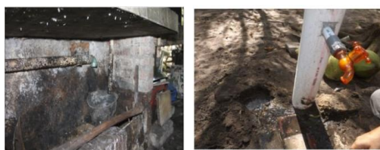
Fig. 4. The wastewater from restaurants' kitchen and hand washing are directly released to the ground
