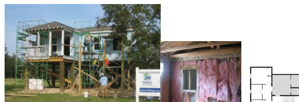
Figure 7. Prefabricated Cottage Expansions by Habitat for Humanity Bay Waveland (above) and stick built expansion by Habitat for Humanity Gulf Coast (below).
