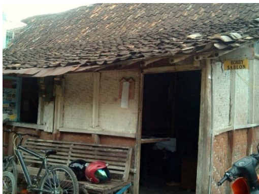
Fig. 1. Sub-standard shelter of poor HBE Source: Field Survey, 2014
