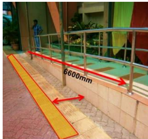
Figure 23: Unsuitable length of the ramp and guiding blocks
