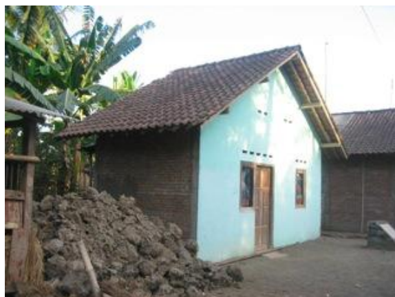
Figure 11. A core house built in Tlogo, Kebon Agung remains in its initial unexpanded form)
